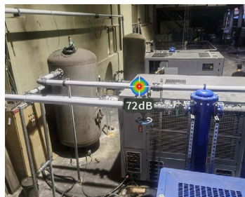
Vacuum System Leaks
