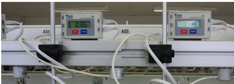
OPS 500 in Meter Handling System
