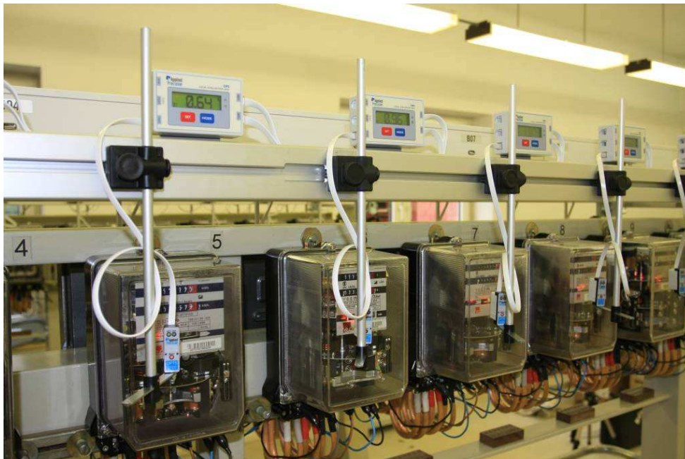
OPS 400 in Meter Handling System
